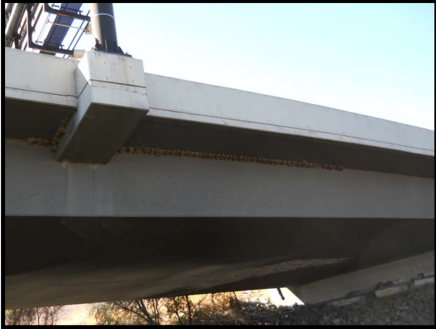
Photo 9 — Looking at the US 6 Bridge over the South Platte River, cliff swallow nests are visible on the bridge
