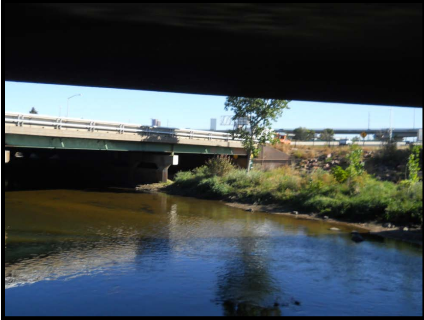
Photo 5 — Looking east from under the US 6 exit ramp to I-25 on the west bank of the South Platte River (Data Point SE-1 in Appendix 4)
